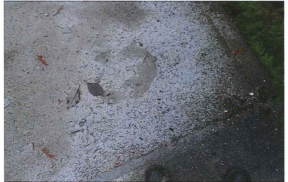
CK2122 Deck Joint
