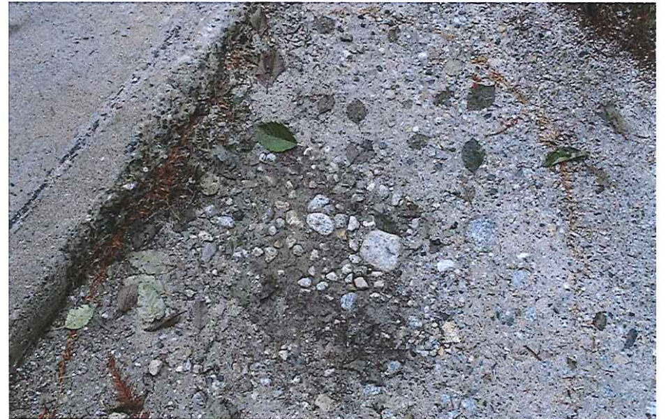
CK2122 Right approach pothole
